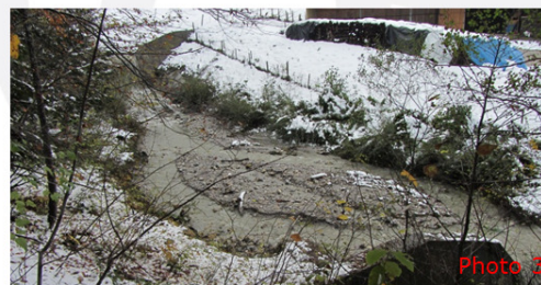
Two sediment / check dams
