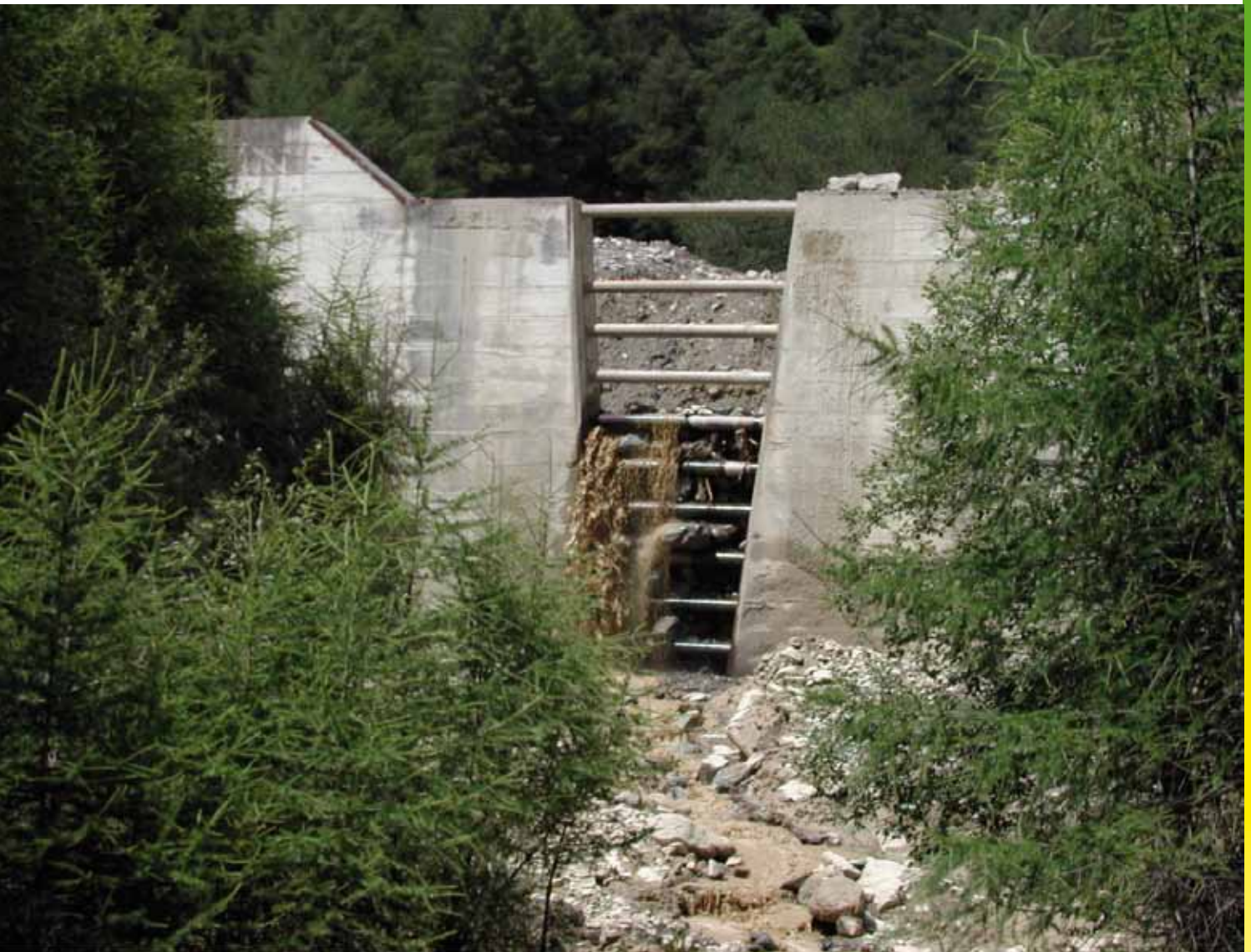
Figure - 7. View of the retention check dam (Gadria stream, NE Italy). Sediment continuity is clearly interrupted; significant costs arise on event occurrence to clean the available retention volume.
