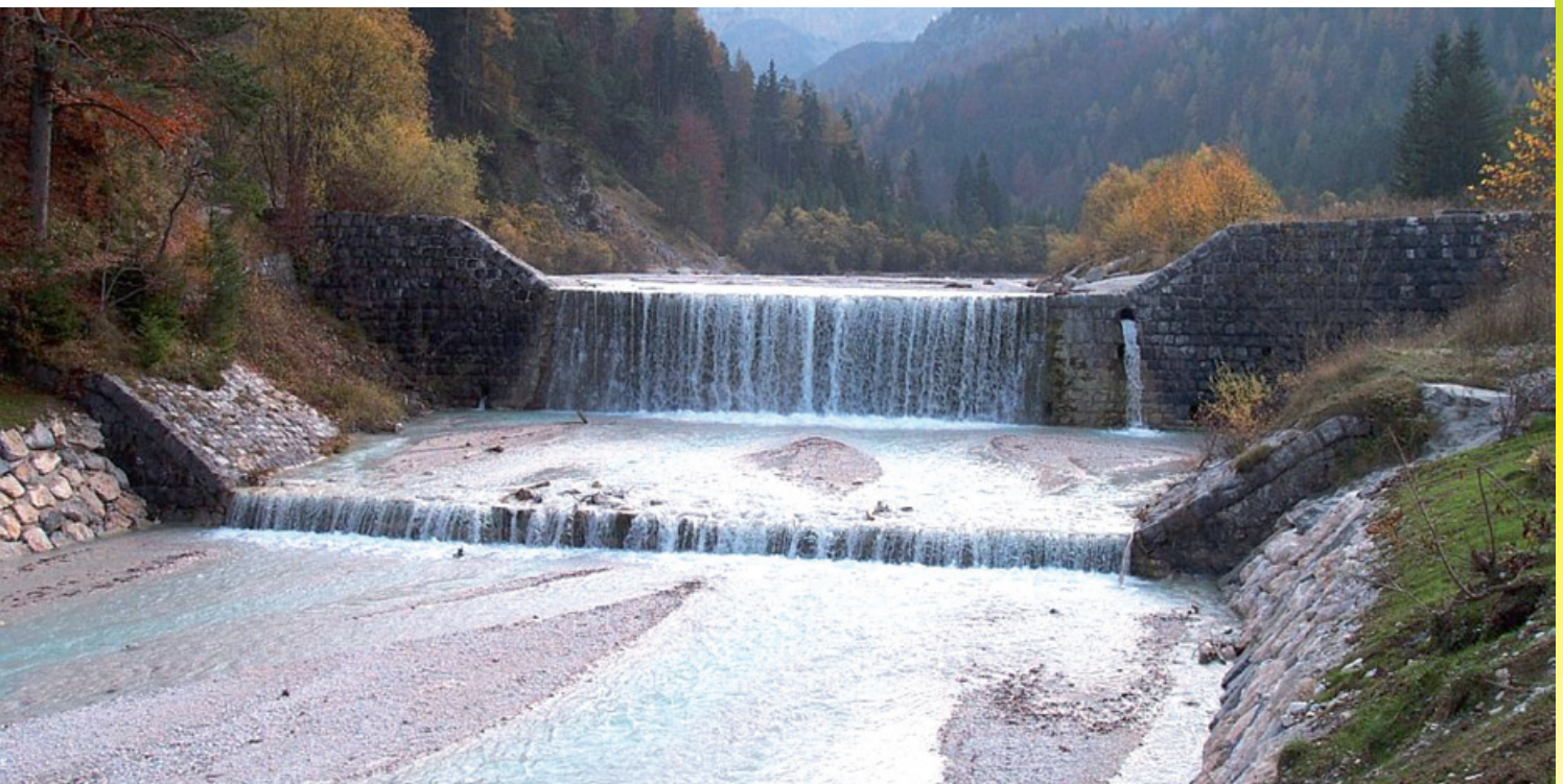
Figure 6 - Check dam on Pišnica torrent in Kranjska Gora (Alpine Ski Center - Slovenia).
